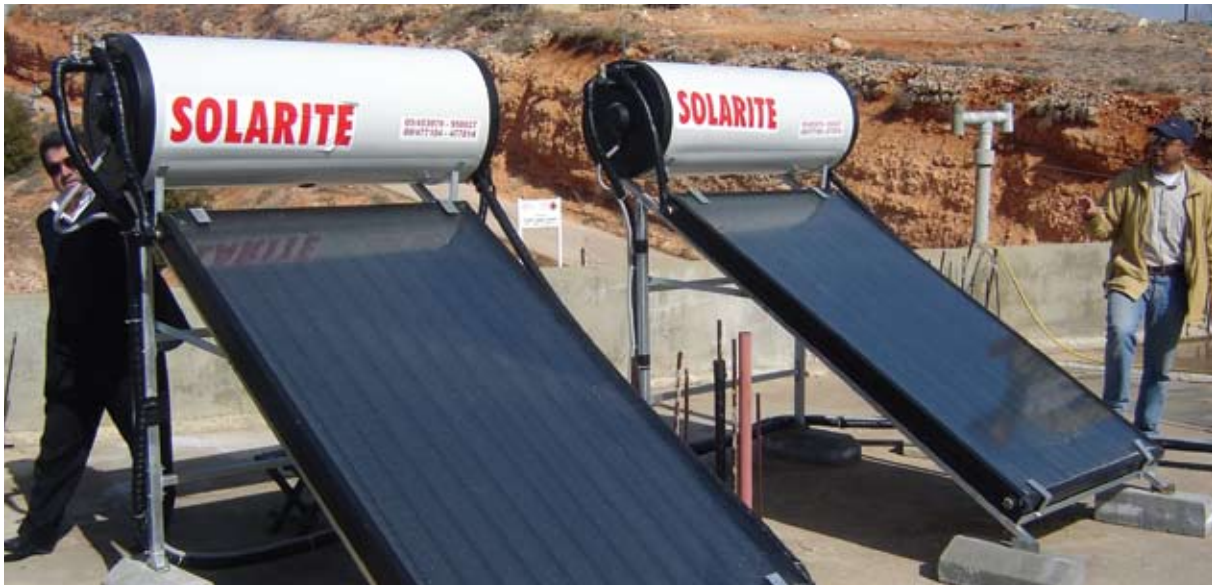
solar water heaters - South Lebanon
